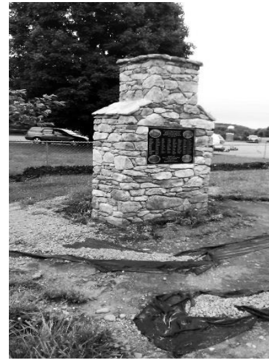
Flood damage by the chimney
